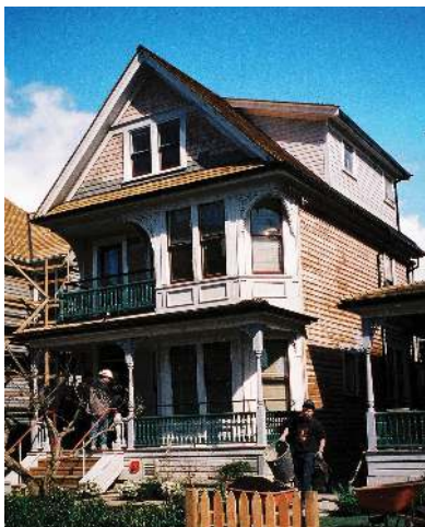
1157 - 1169 Pendrell St Mole Hill Restoration of lost Victorian detailing on four houses including Paterson House , 2003 Heritage Register: B
