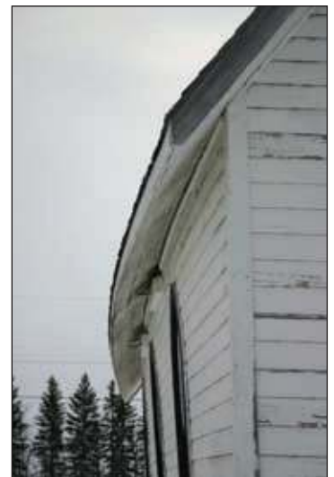
Bowing of an exterior wall, likely due to foundation issues, will eventually collapse if not repaired.
