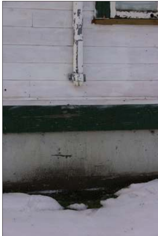
With a missing downspout and inadequate grading, water is allowed to collect at the base of the building and can cause significant damage.
