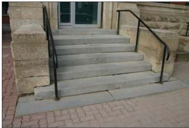
These steps need to be inspected as the freeze/thaw cycle is causing some lifting. A mason may have to re-level them.
