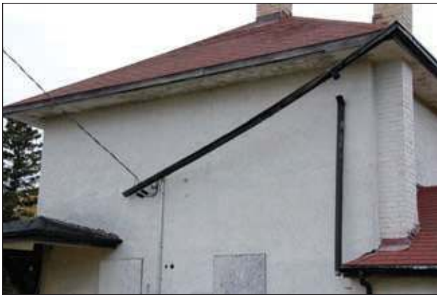
The gutter has fallen off, onto a power line. This is now more than a maintenance issue, but a fire hazard.
