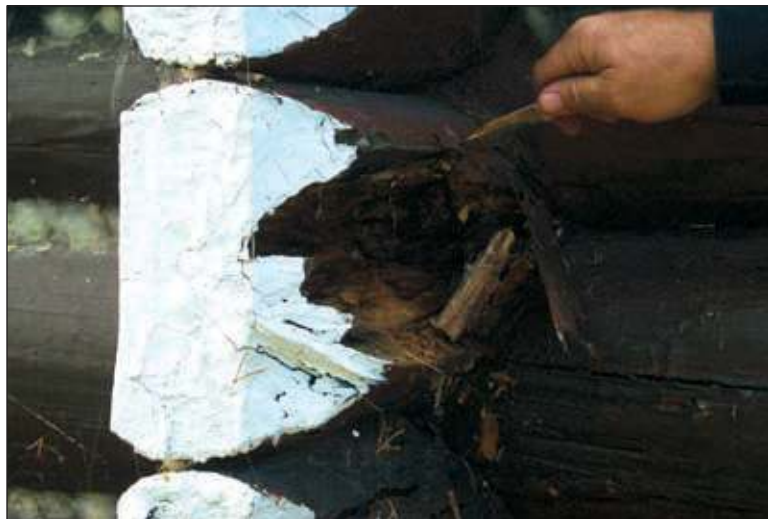
This log has been damaged by water. Investigate the source of the water and address the cause of deterioration before replacing the log.
