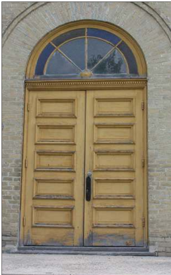
This door needs a new coat of paint to retain the original integrity. The weatherstripping should also be inspected.
