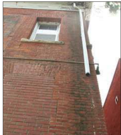
The missing downspout has created a build up on the exterior wall. Cleaning may do more damage, so it may be better to just leave it there.
