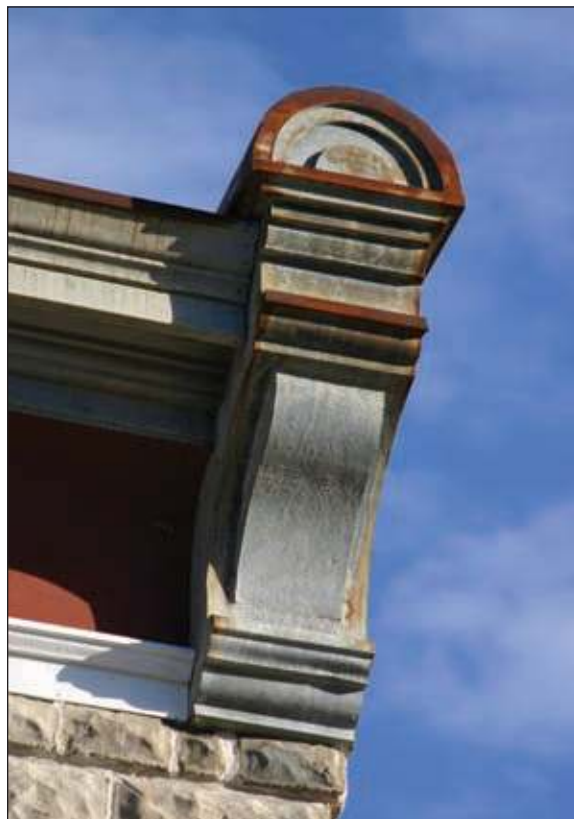
This eave bracket needs to be painted to prevent further deterioration by rust.
