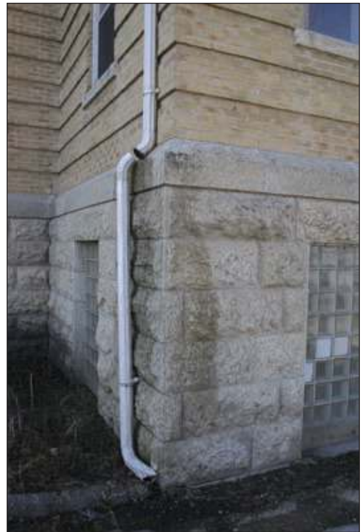
This downspout has come detached between the first and second floors making it completely ineffective. Also it is missing a leader to direct the water away from the building, which would cause foundation damage.
