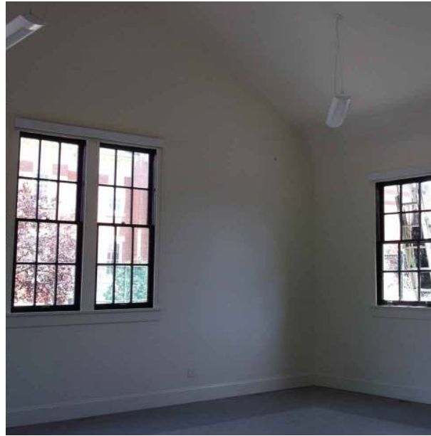
■ Left: Carleton Hall's interior prior to rehabilitation, with part of the roof missing and fire and water damage
