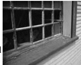
Photo: Damaged Window Sill
